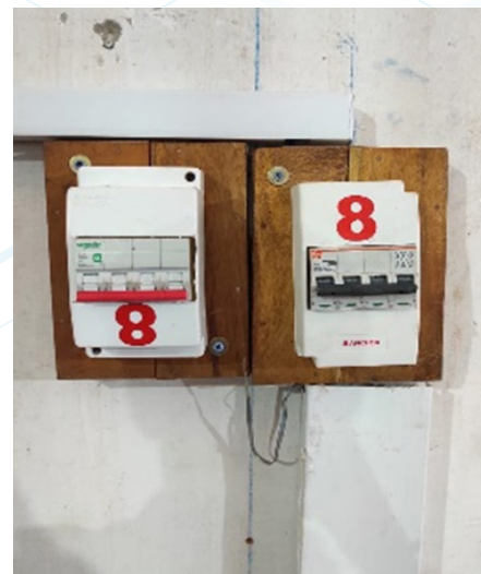
Providing individual MCB Switches to each Machine
