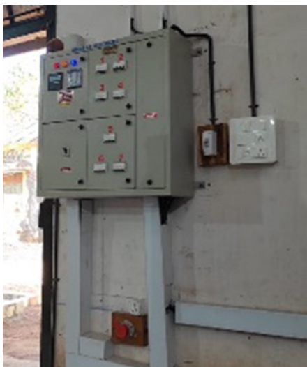
Main Control Panel Box
