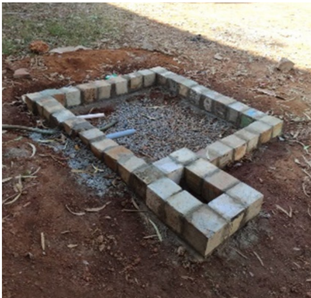
Earthing for Electric connections
